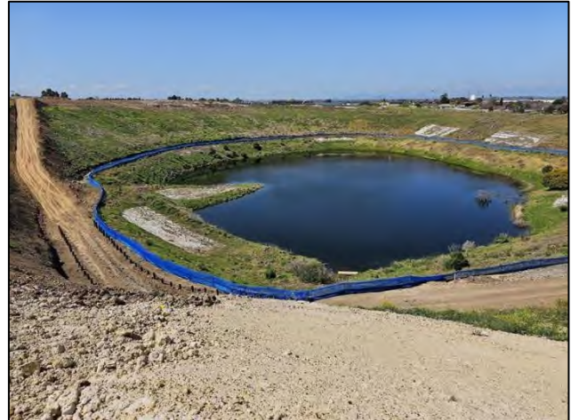
Plate 2. The north west area of offset area where backfilling and piling undertaken (Ecology and Heritage Partners Pty Ltd 26/09/2023).
