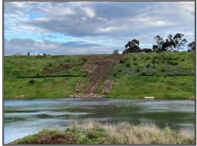
Plate 8. Rock beaching and habitat improvement works underway in offset area 1 (site 1) (Ecology and Heritage Partners Pty Ltd 26/04/2022).
